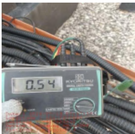
BAR GROUNDING TOWER
