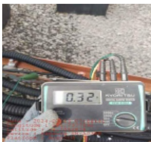
IGB / INDOOR SHELTER
