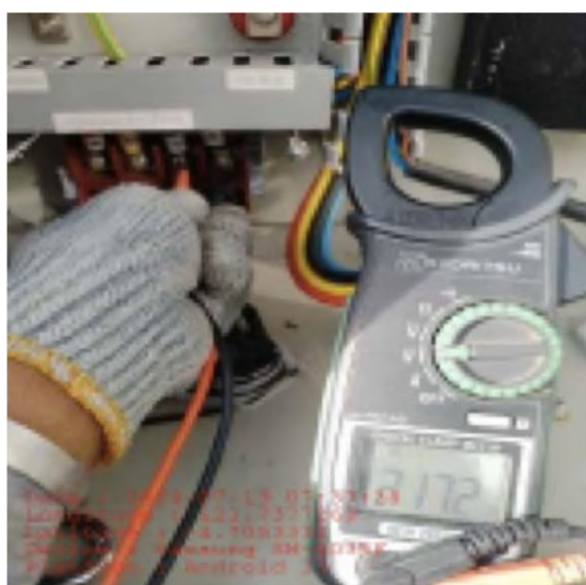
PENGECEKAN PHASE VOLTAGE
